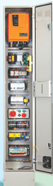
MRL Control Panel
